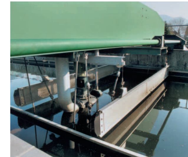
Returned sludge pump installed on a rotating scraper bridge.
